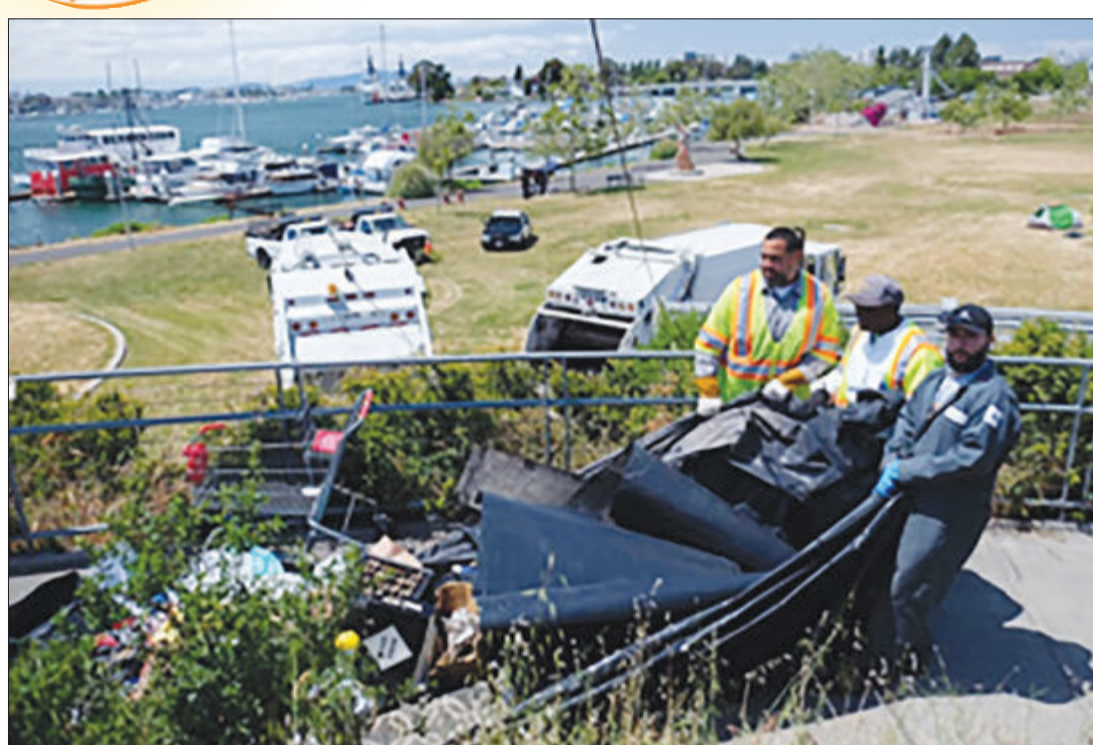
Workers from the City of Oakland clear debris from the hilltop at Oakland's Union Point Park directly across the Oakland Estuary from Alameda. Brock de Lappe
